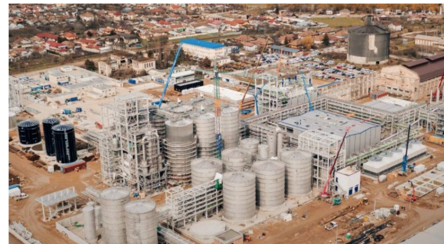
Clariant's bioethanol plant @ Romania
